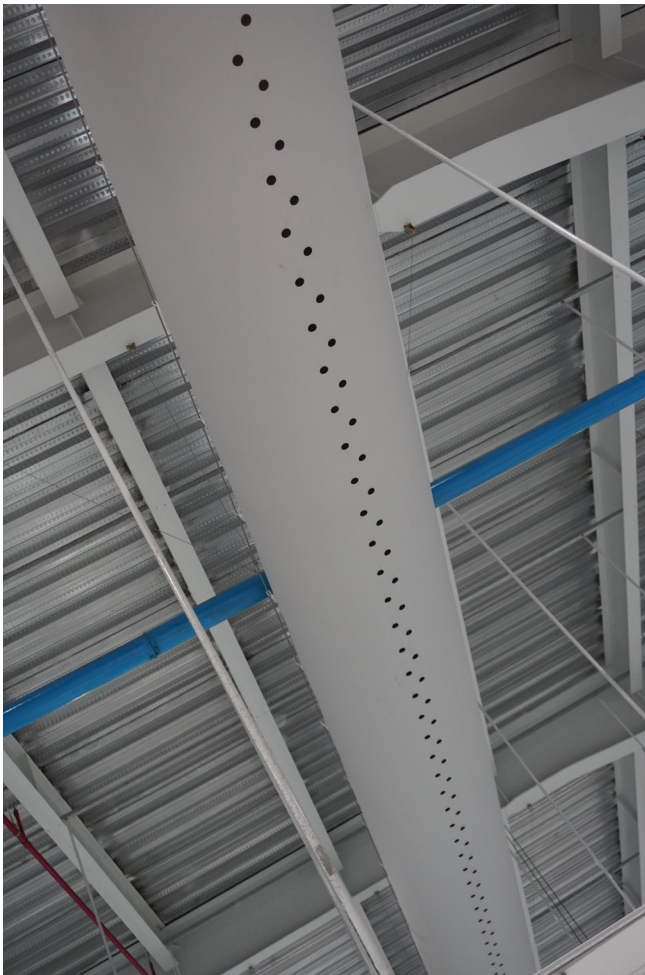
View of fabric air dispersion ducts. Image courtesy of WorldOn.
