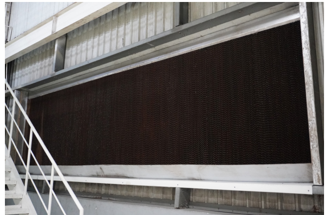
External view of a water curtain at the factory. Image courtesy of WorldOn.
