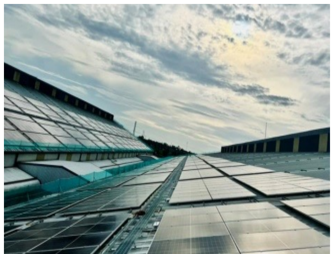
Solar array on the roof. Courtesy of An Giang Samho
