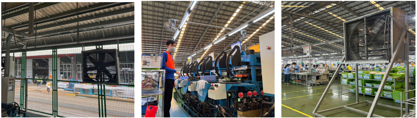
Interior images of exhaust and worker station fans. Courtesy of An Giang Samho
